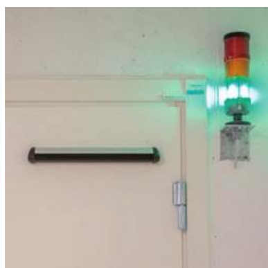
Signal tower outside collection room
