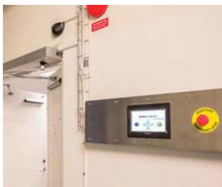
Control unit installed on the wall
